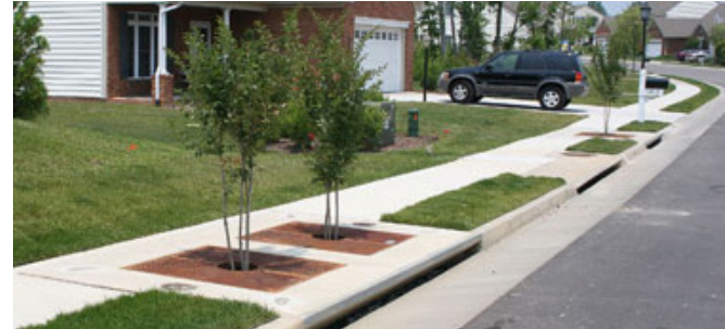
Tree box for stormwater treatment in boulevard
