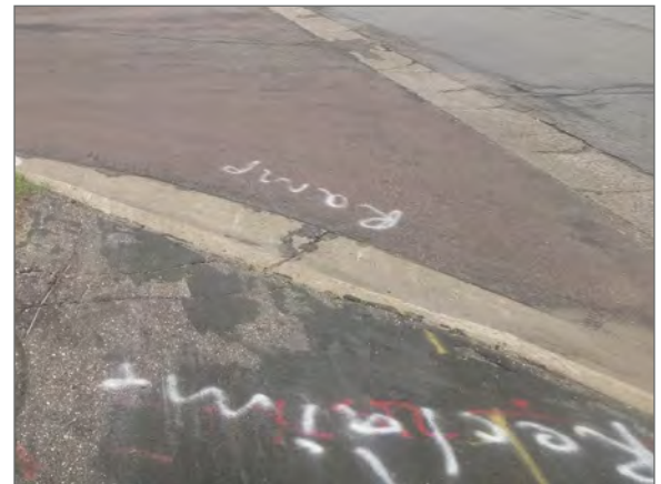
Improvement to be completed on a sidepath along Anderson Lakes Parkway in Eden Prairie.
